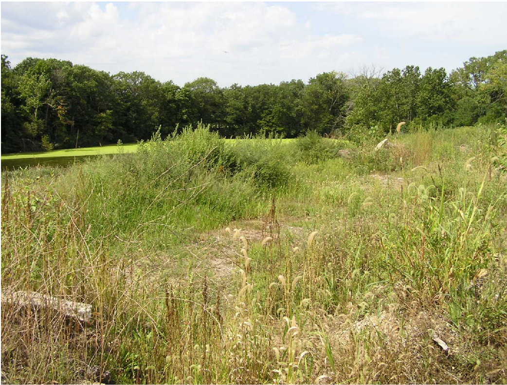
Date:09-04-2014 Time: 12:42PM Direction: Northwest Photo by: Jen O'Hearn Exposure #: 011 Comments: View of water and piles along the edge of excavation.
