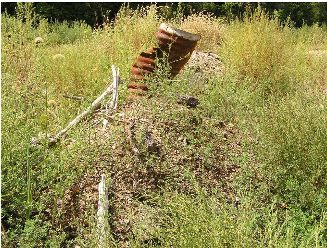
Date:09-04-2014 Time: 12:32PM Direction: Northwest Photo by: Jen O'Hearn Exposure #: 006 Comments: View of corrugated metal pipe in with a soil, rock, asphalt pile covered with weeds.
