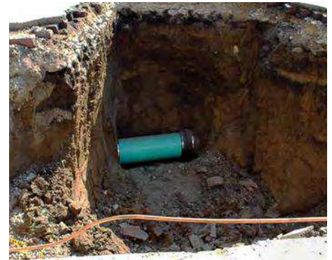
Bloomington Public Works takes a proactive approach to sanitary sewer, stormwater and water infrastructure maintenance, ensuring underground infrastructure is repaired prior to roadwork. (Photo provided)
