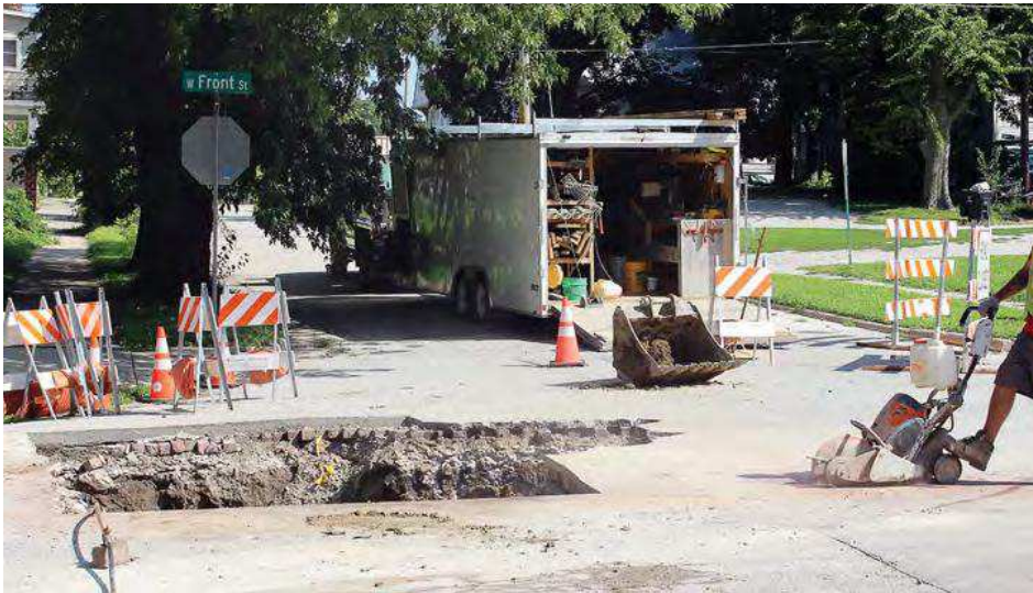
A public works employee cuts into the street as part of a sewer dig. (Photo provided)
